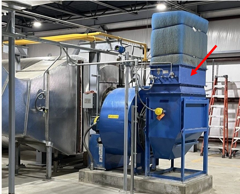
Photo No. 1: Combustion Air Flow Meter
